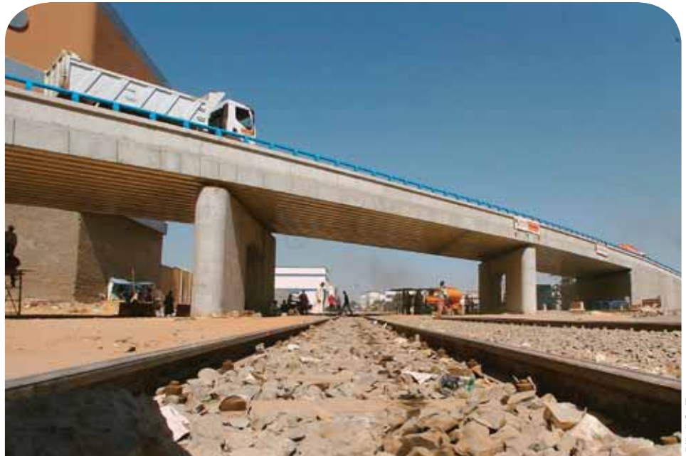
Construction in Dakar, Senegal: IMF–World Bank debt issuance plan includes focus on bond financing for African infrastructure.
